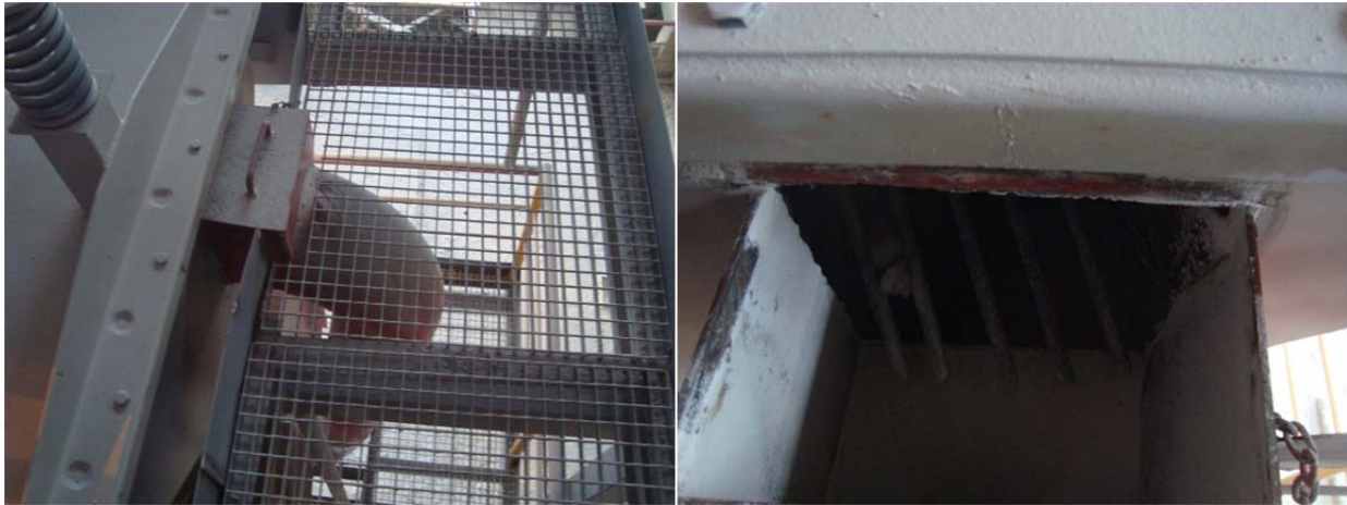
Fig. 9 – Device for lumps removal from vibrating feeder
