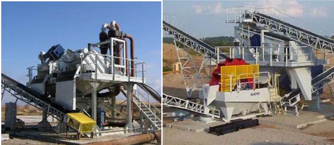
Fig. 11. Sand Recovery System: left Hydro Cyclons in combination with Dewatering Screens, right Bucket Wheel
