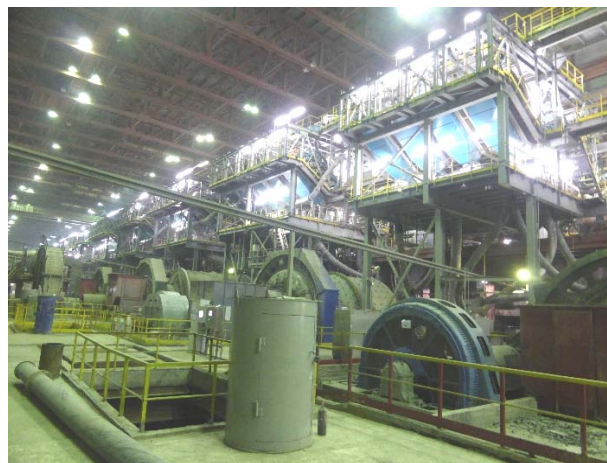
Fig. 1. The crushing unit at ANOF-3 after revamp
