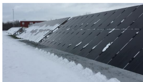
Fig. 1. Experimental PV-panels of the Regional Test Centre in Williston (Vermont, USA) with frameless (foreground) and traditional (in the background) modules for studying the effect of snow on electricity generation and the bearing structure of PV-panels
