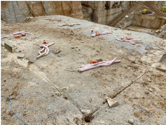
Fig.11. Pre-cutted along the perimeter block of overburden, repaired for loading with explosives.
