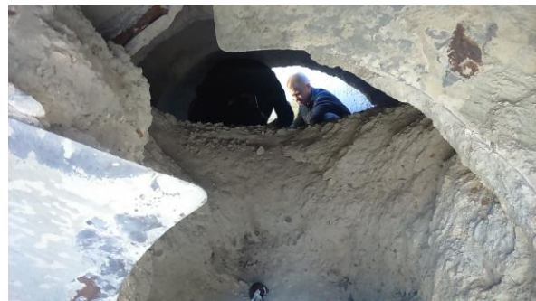
Fig. 3. Concrete mixer interior
