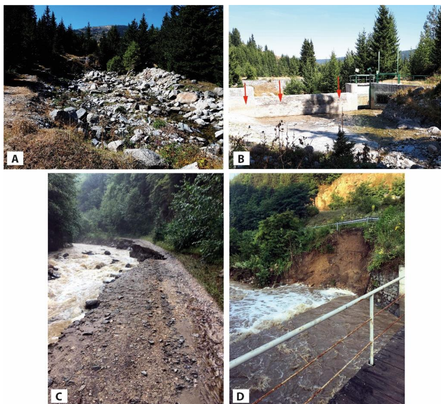
Fig. 2. (A) Deposition related to mid-2019 flood event just above the water intake for the Belmeken dam. Photo taken in September 2019. (B) The water intake weir for the Belmeken dam. Stains related to the accumulation of wet sediments are marked with red arrows. (C) The main river channel side erosion. The main access road for the Cherna Mesta catchment, above the power plant. (D) Partial collapse of road II-84 (Velingrad – Razlog). Photos (C) and (D) were taken on 23 July 2019 and were provided by the Yakoruda municipality.
