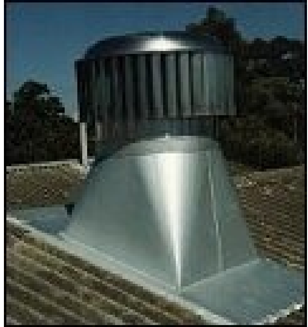
Figure 4. Outside view of turbine fan
